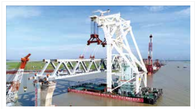
孟加拉国“梦想之桥”——帕德玛大桥架设主桥钢梁 Main bridge steel beams were erected on the “Bridge of Dreams”, the Padma Bridge, in Bangladesh
