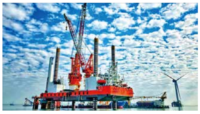
福清兴化湾海上风电场一期项目 Offshore wind farm phase I project in Xinghua Bay, Fuqing
