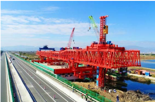
● 中铁工业研发的世界首台桩梁一体架桥机“共工号” “Gonggong No.,” the world’s first pile beam integrated bridge erecting machine developed by China Railway Hi-tech Industry Corporation Limited
