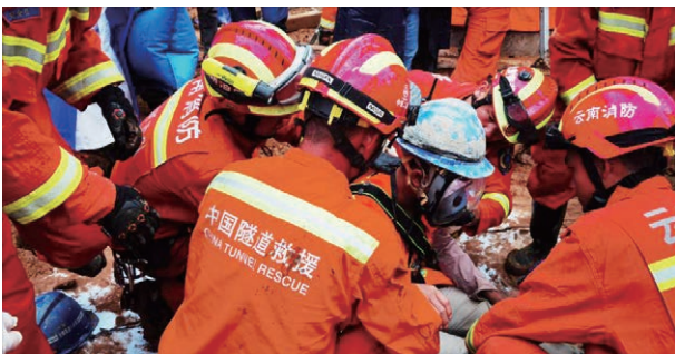
● 中国中铁救援队紧急驰援云南隧道坍塌抢险 CREC Rescue Team rushed to rescue people from the collapsed tunnel in Yunnan
